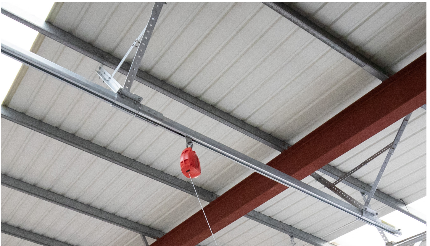
An example of a finished parallel installation.
